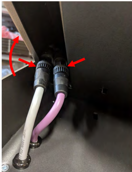
Figure 16-28 Power and Communication Cables
