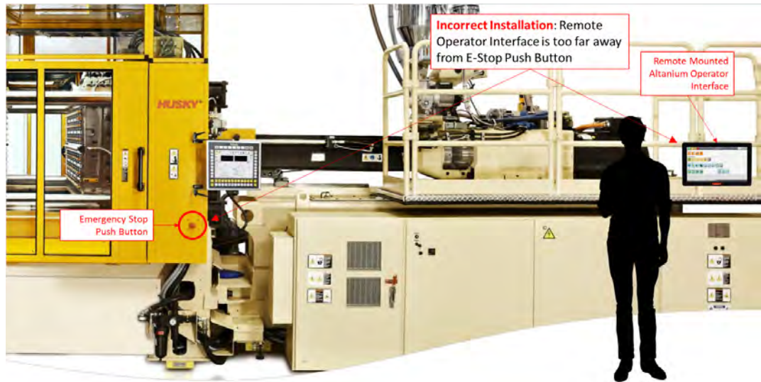
Figure 2-9 Incorrect Installation Position of Remote Operator Interface
