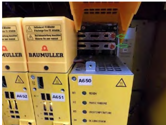
Figure B-3 DC Bus Bar Under Cover
